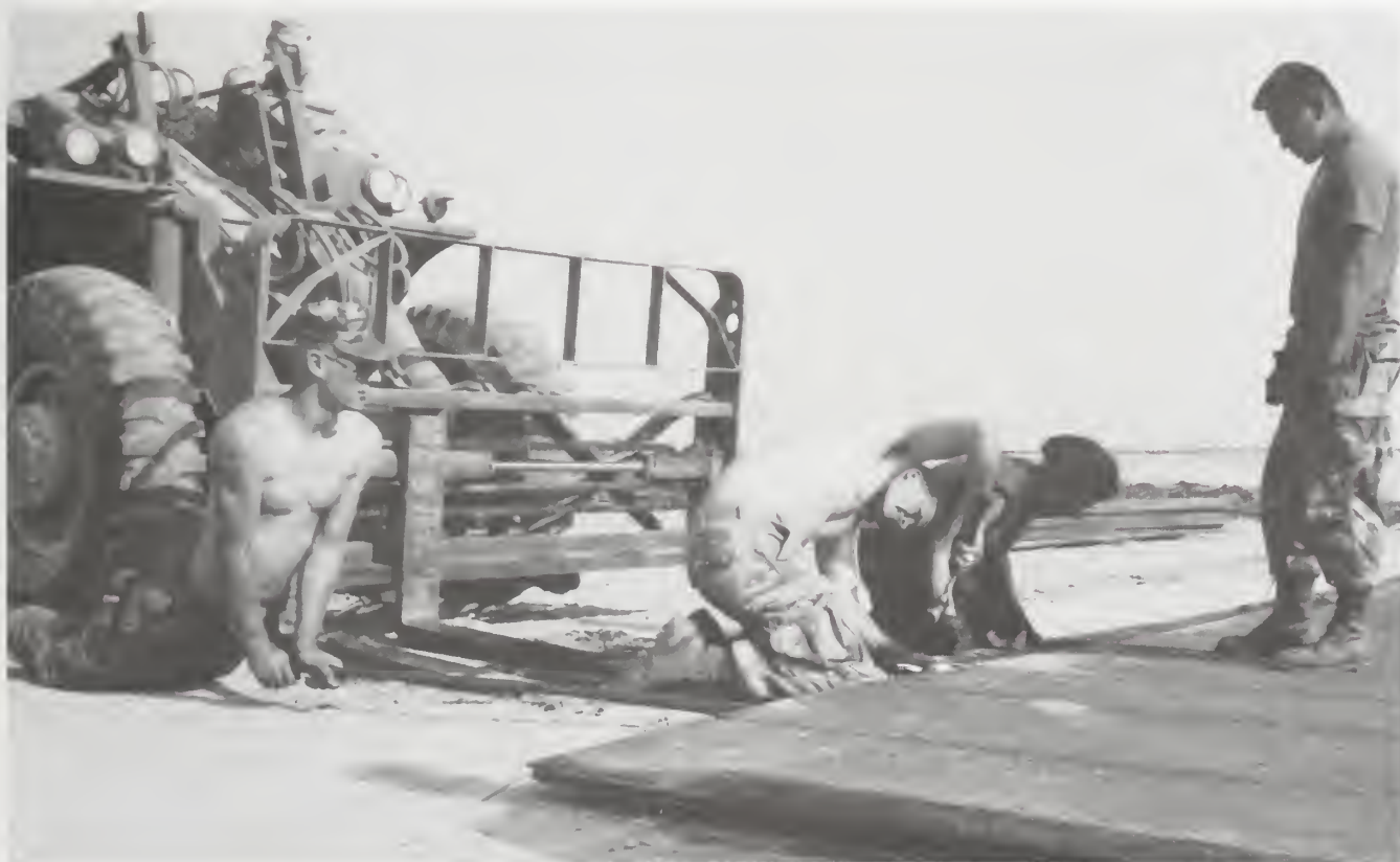
Marines from MWSS-271 lay aluminum matting for an expeditionary airfield at Tanajib, Saudi Arabia, 1991.
